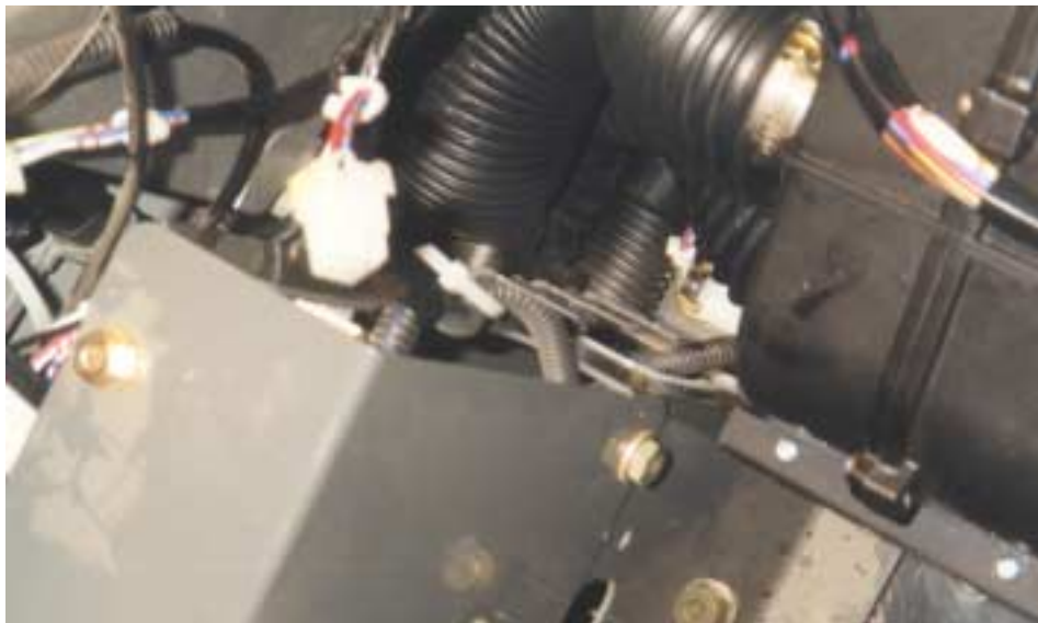
Flex hoses connecting to the forward air duct.
