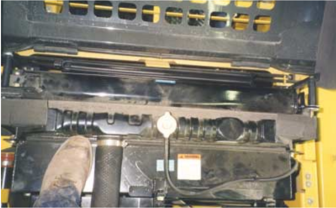
Top brackets on condenser frame showing spacers in place.
