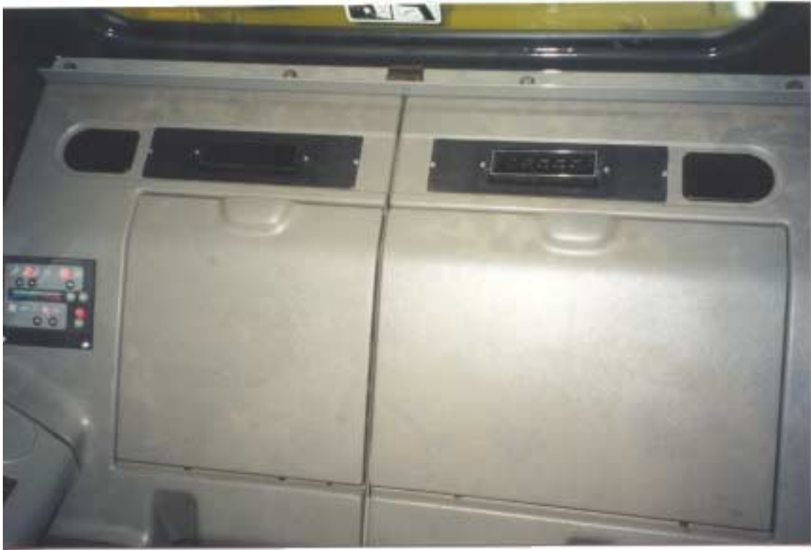
Louvers and controls in place.
